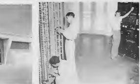
Ready for action this weekend is the new Telephone Exchange (above). There will be minimum interruption of service while the switch-over is made. Here's how the switch will be made: Marciano Arends, right, closes the main fuse; Marciano Arends (center) clips wires, and Victor Winterdaal, left, pulls out
